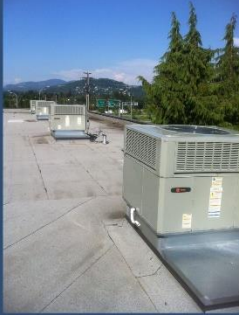
28 HVAC roof top units
